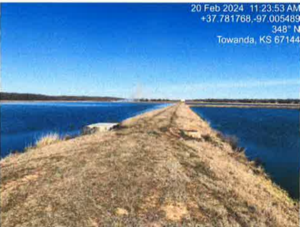
Photo Taken: 2/20/2024 11:23:53 AM Looking at all cells (Cell 1 left, Cell 3 right, Cell 2 background upper right).
